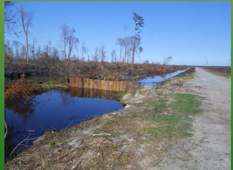
Temporary check dam, Interior Ditch, during Lateral West Fire, GDS NWR, by L. Mitchell.
